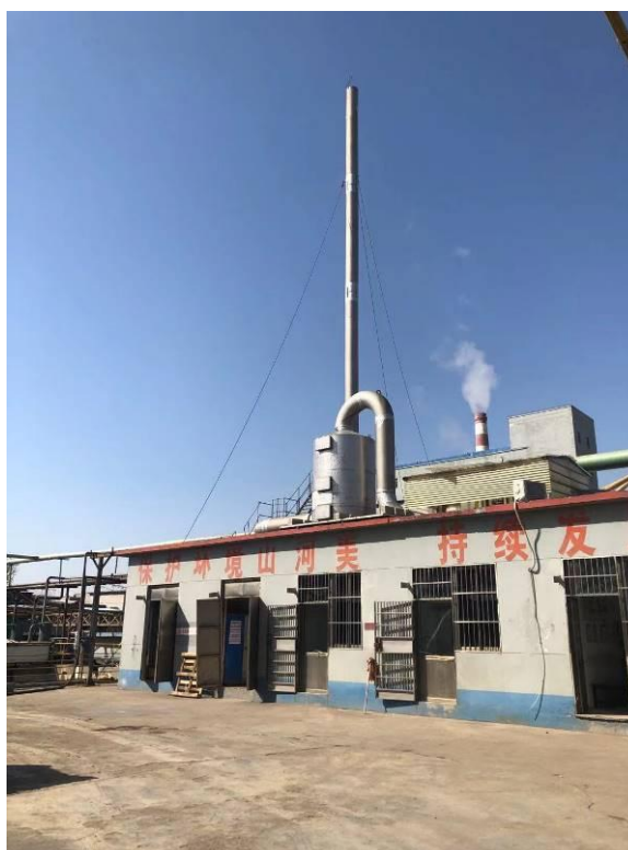
污水站臭气排气筒 (h=30m/r=0.6m)
